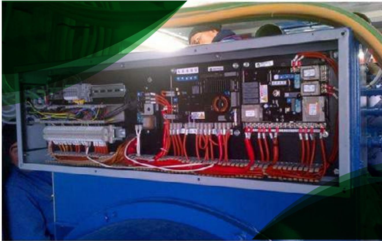
Above: the control unit, for Biogas project of Cerignola.
